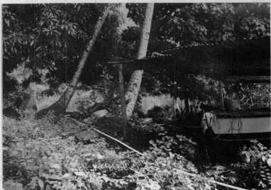
Figure 5. Piping from pump to Epinup Village.
